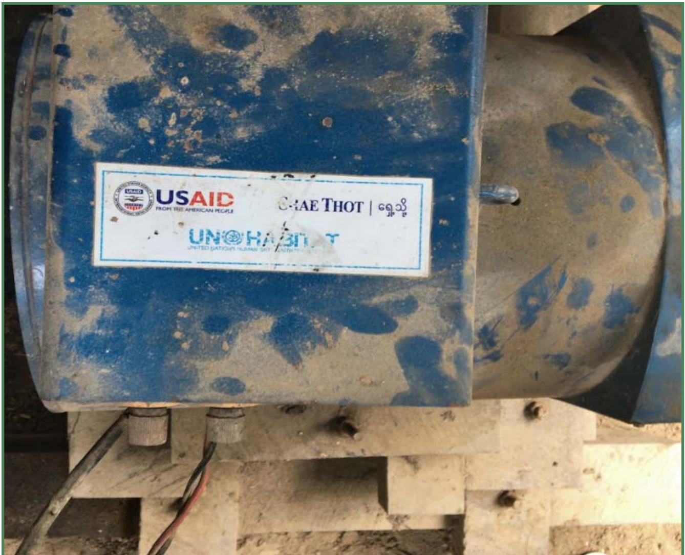
A dynamo connected to the generator (DMG setup) in a village in Seikphyu
