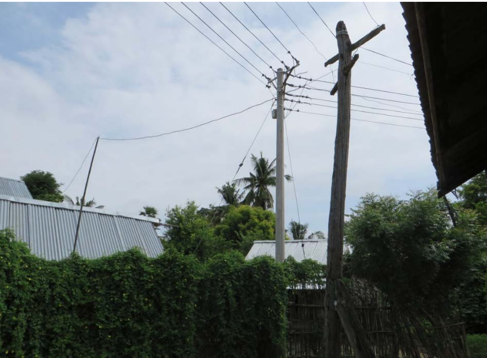
Old DMG setup (wooden poles) and new LT grid setup to connect to the national grid in Ah Mhu
