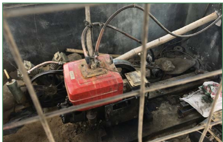
Diesel Generator in Than Pyar Pin
