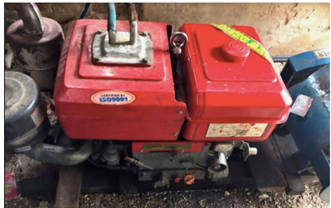
Diesel Generator in Kone
